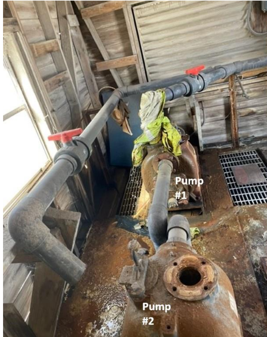
Lift Station 1151 – only one pump is hooked up and operational. handles industrial waste from CCAD Building 8, Building 340 and other CCAD industrial facilities.
