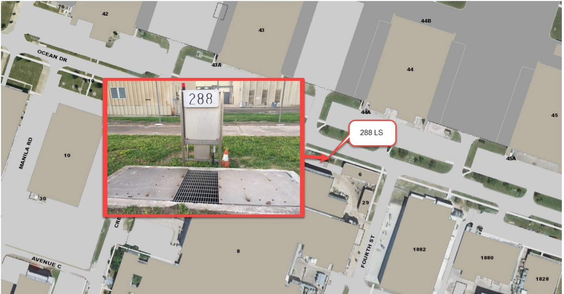
Lift Station 288 – Underground storage of domestic wastewater from Corpus Christi Army Depot and several Naval Air Station Corpus Christi tenant command buildings.
