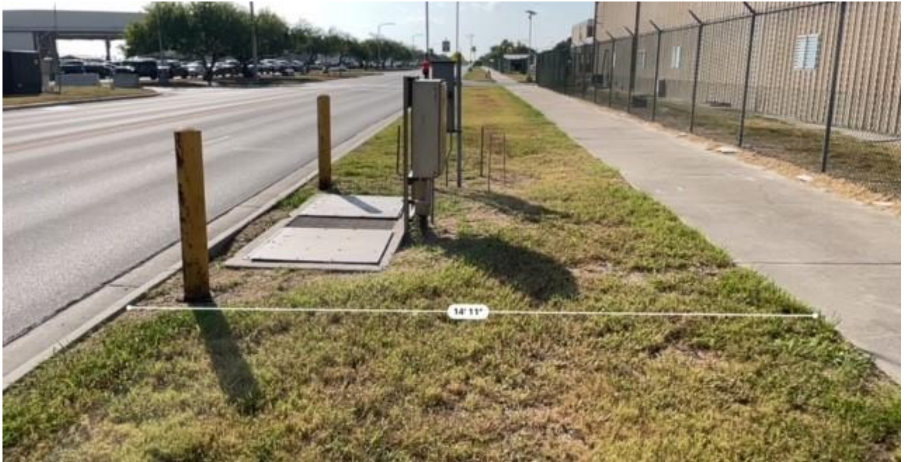
Lift Station 288 was built in 1978. It contains two submersible grinder pumps. Only one of the pumps is functioning. Its capacity is one million gallons per day (1 MGD).
