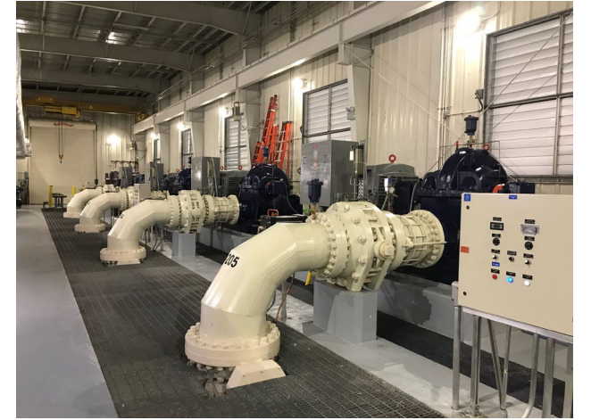
Woodsboro Pump Station
