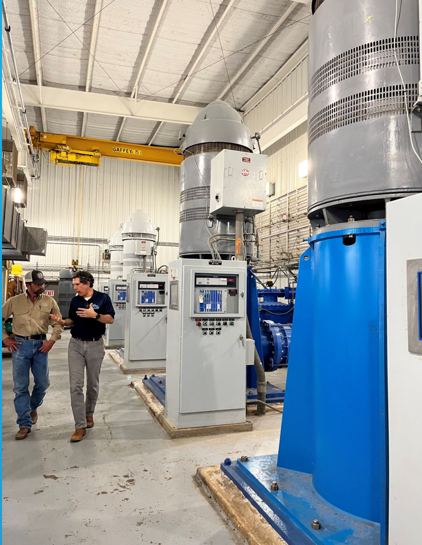
LNRA Intake Station
