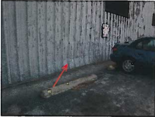
Cladding Damage @ Ocean Air Center
