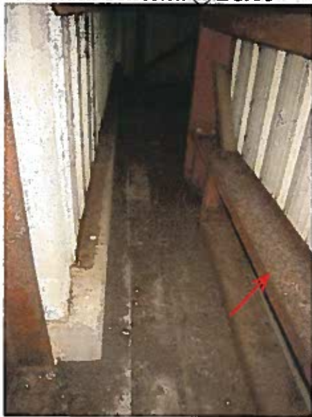
Door Pocket Corrosion @ EGA 3
