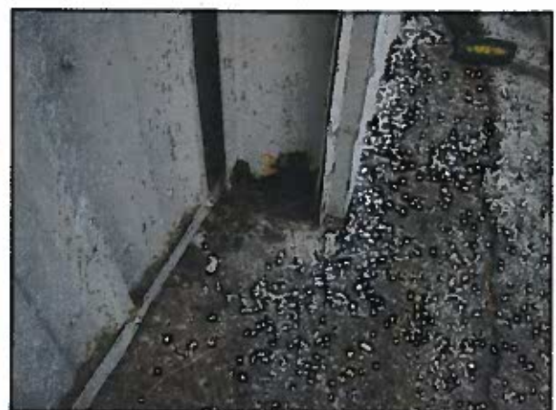
Severe Corrosion Damage @ OAC Doors
