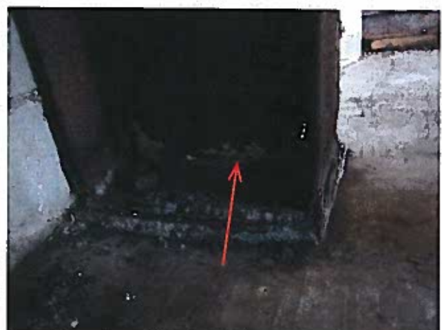
Severe Corrosion Damage @ EGA 3 South Wall
