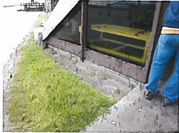
Poor Drainage @ SWA Storefront
