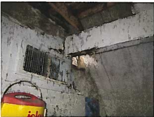
Water Damage to Walls and Wood Framing
