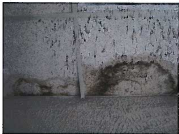
Water Damage to Ceilings
