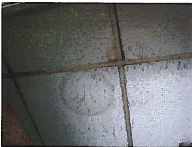
Stained Ceiling Tiles @ Dodd Aviation - 1
