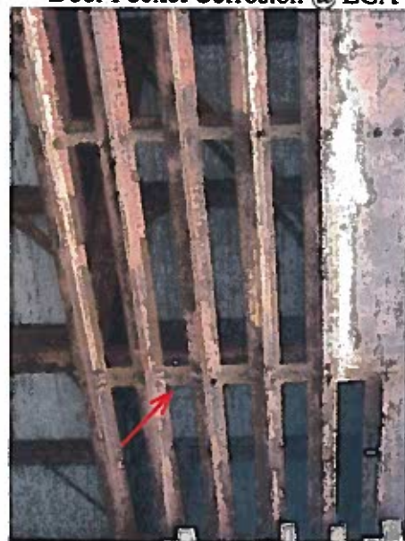
Upper Door Track Corrosion @ EGA 3
