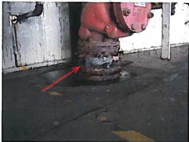
Fire Sprinkler Riser Damage @ EGA 3
