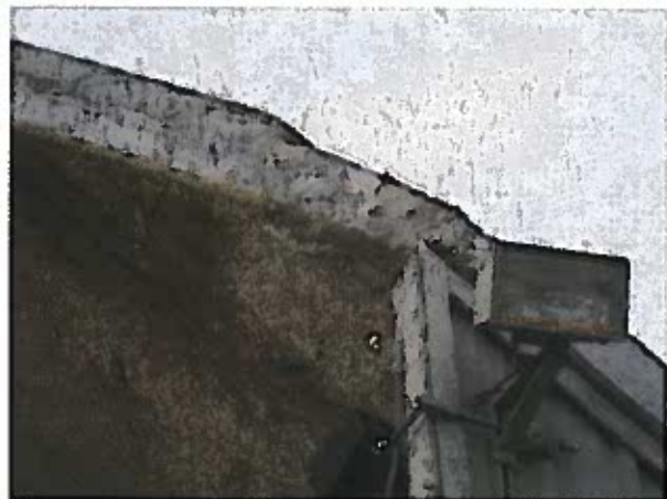
Exterior Spalls – Previously Patched
