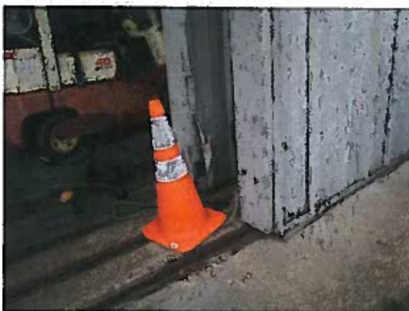
Door Damage @ OAC
