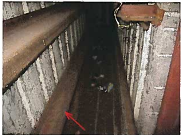
Door Pocket Corrosion @ EGA 3
