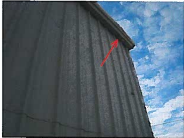
Missing Downspout @ Ocean Air Center
