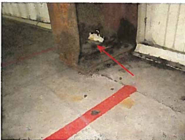
Severe Corrosion Damage @ EGA 3 South Wall
