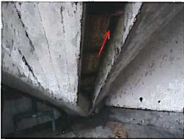
Fiberglass Infill w/ Rotted Framing
