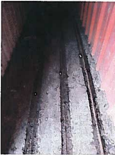
Corroded Door Tracks @ OAC
