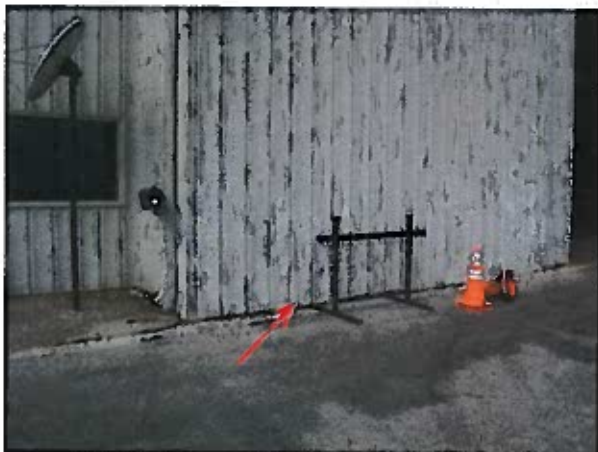
Panel Damage @ EGA 3
