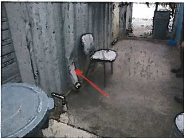
Downspout Damage @ Ocean Air Center
