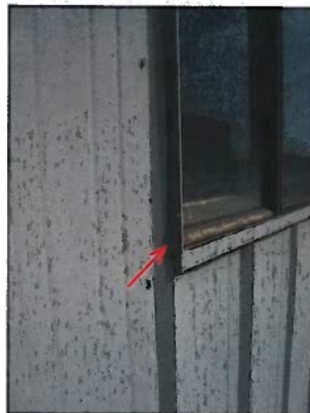
Caulking Around Windows is Missing
