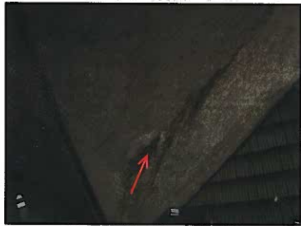
Water Infiltration w/ Spalling
