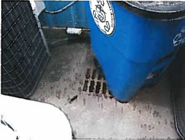
Partially Blocked Drain @ OAC
