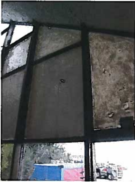
Damaged Glazing @ SWA Cargo
