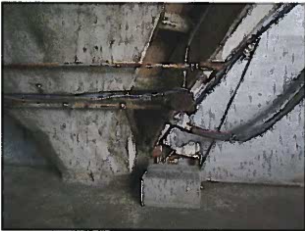
Water Damaged Electrical Conduit
