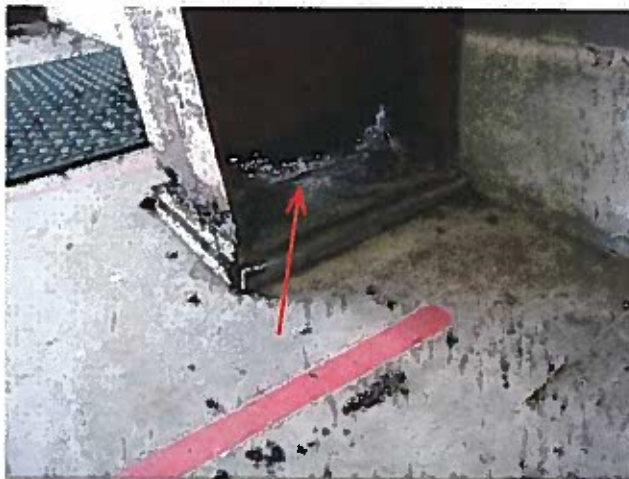
Severe Corrosion Damage @ EGA 3 South Wall
