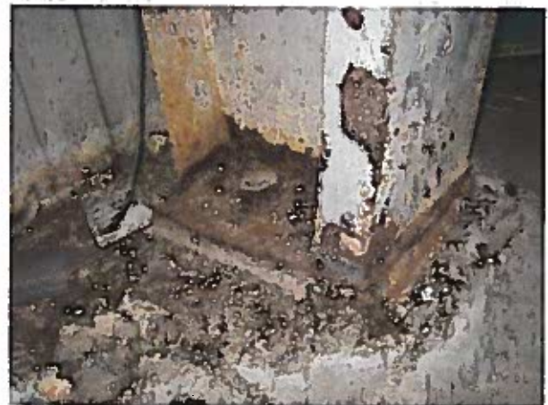
Baseplate Corrosion @ OAC
