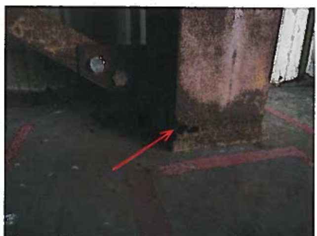
Severe Corrosion Damage @ EGA 3 West Wall
