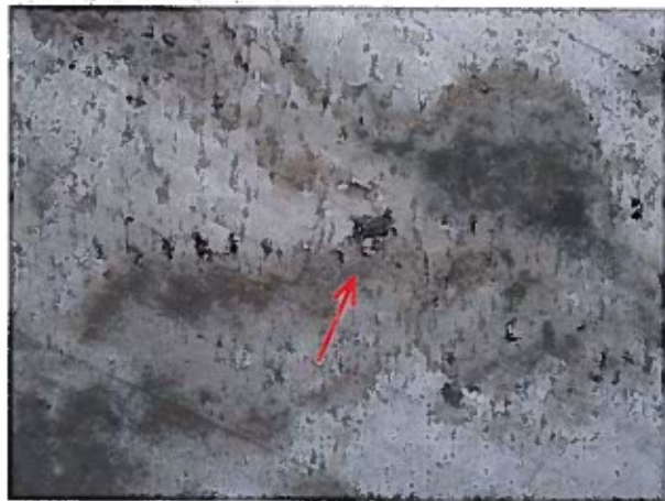
Water Infiltration w/ Spalling
