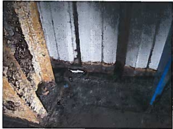
Panel and Base Angle Corrosion @ OAC
