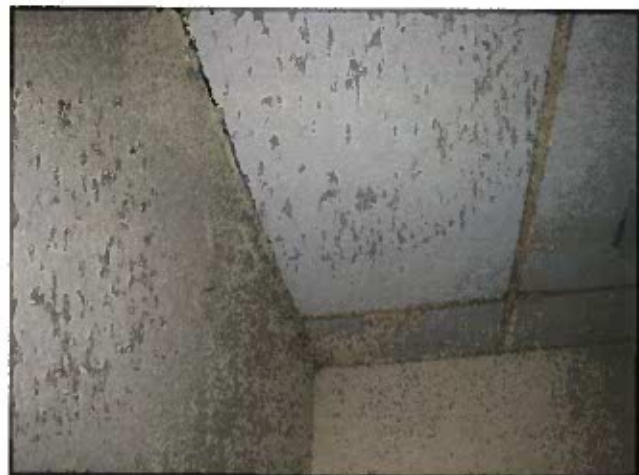
Stained Ceiling Tiles @ Dodd Aviation - 2
