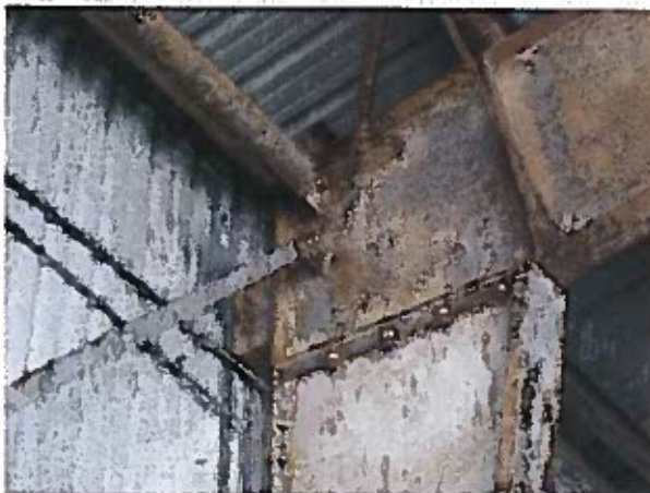
Primary Member Corrosion @ OAC
