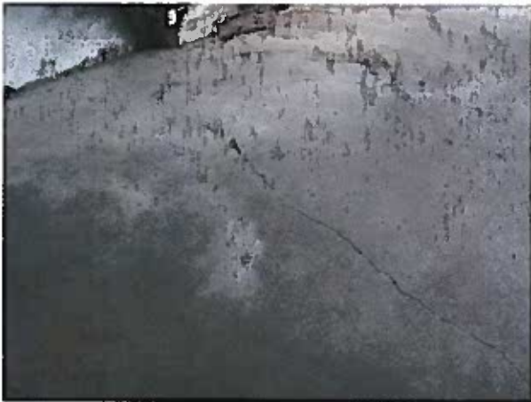
Floor Slab Cracking
