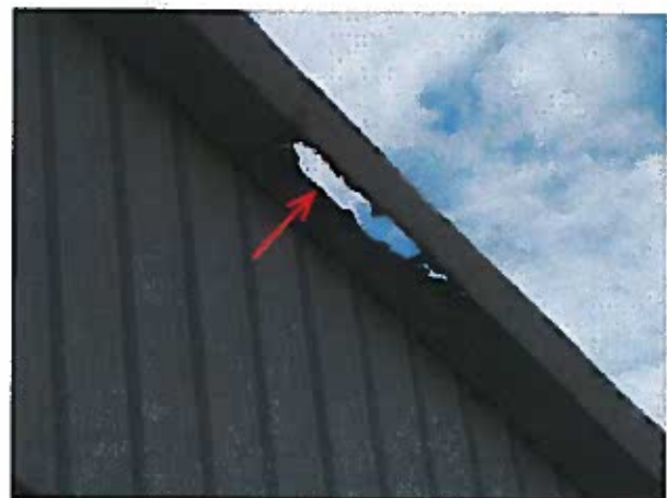
Gutter Damage @ EGA 3
