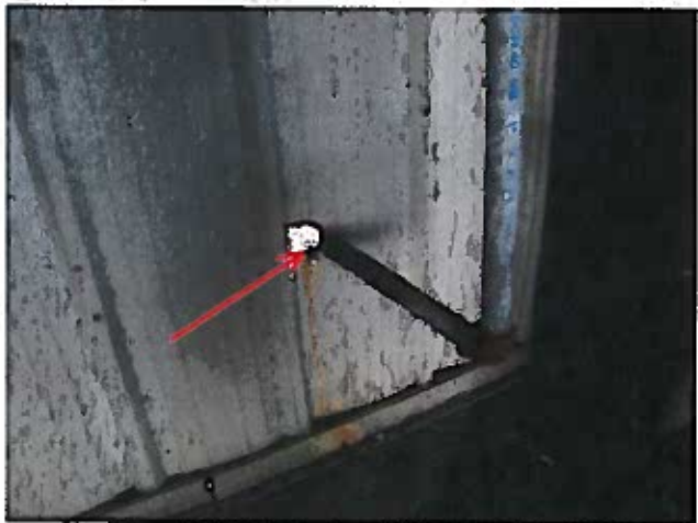
Overflow Corrosion Damage @ EGA
