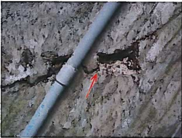
Cracking in Concrete Shell
