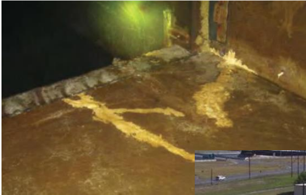
↑ One of many cracks in concrete
