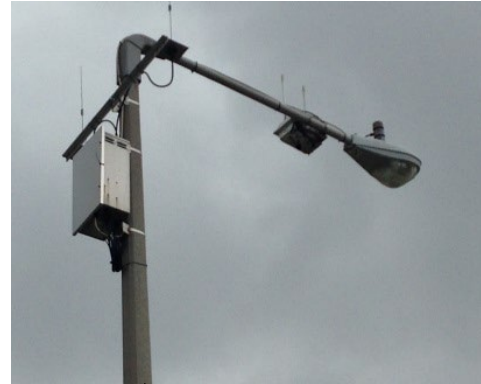
Data Collection Unit (DCU)
