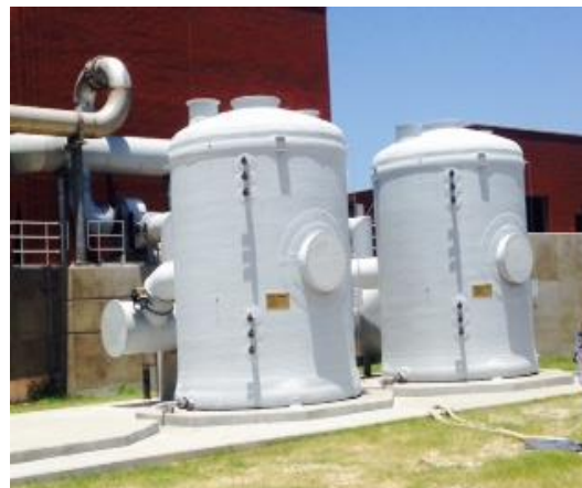
Sludge Odor Control
