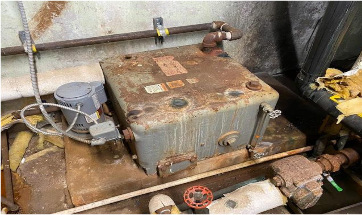
Condensate Return Station #15 – Engine Test Cell Mechanical Room
