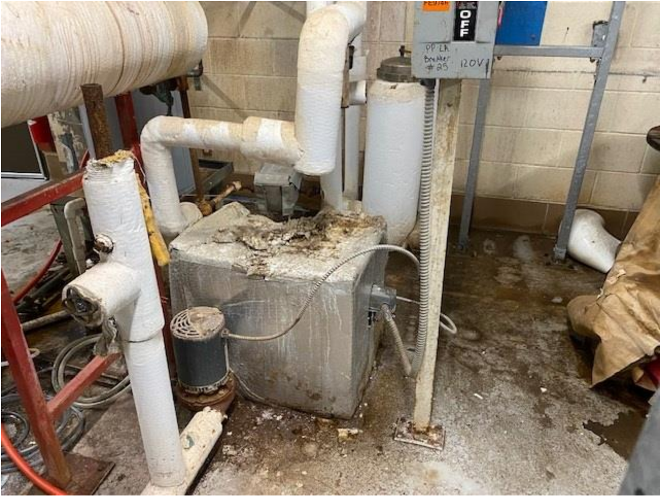
Condensate Return Station #13
