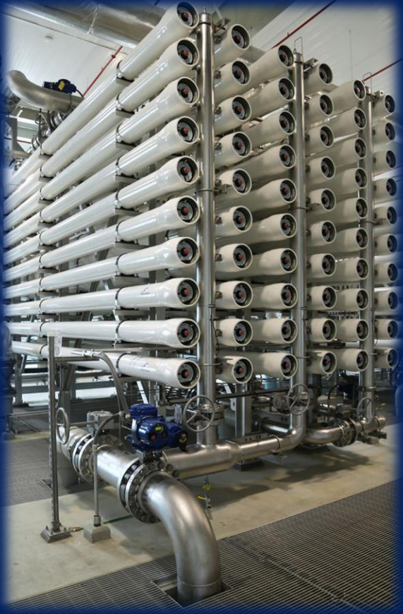
Reverse Osmosis Plant
