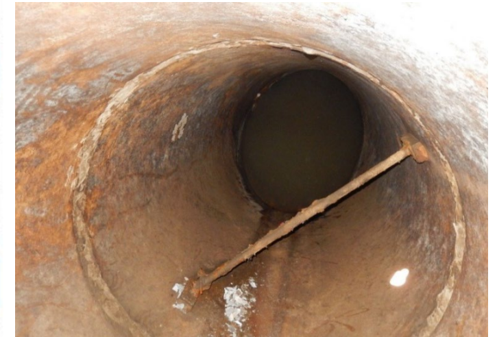
Debris Found in Pipeline
