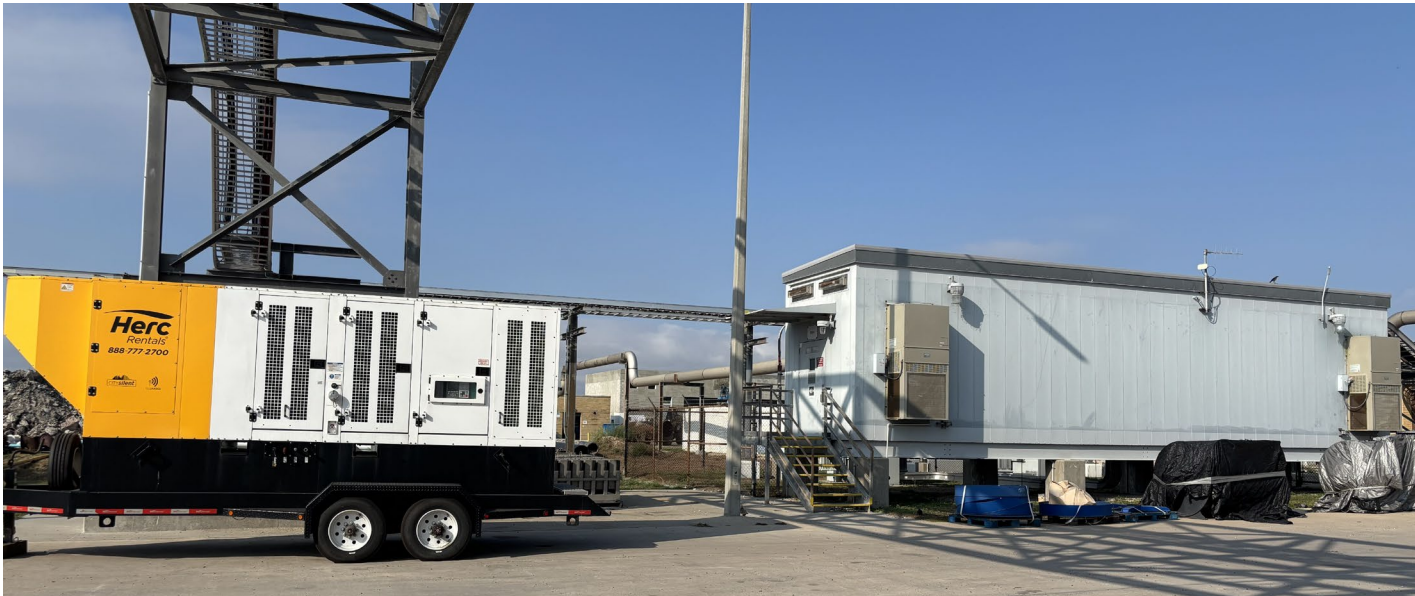
Temporary Generator Rental at the Electrical Control Room
