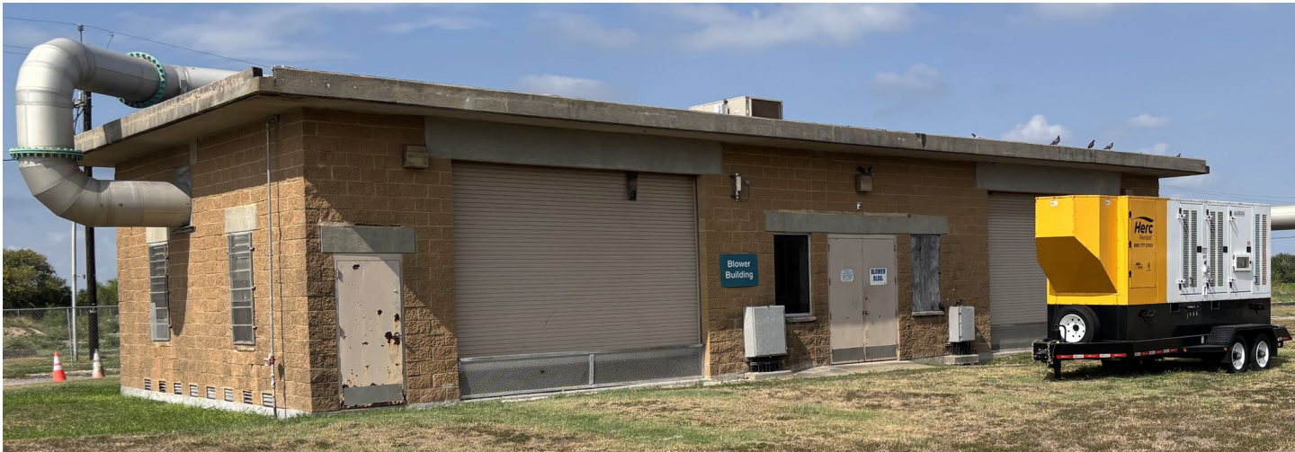
Temporary Generator Rental at the Blower Building
