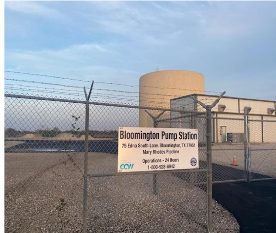
Bloomington Pump Station
