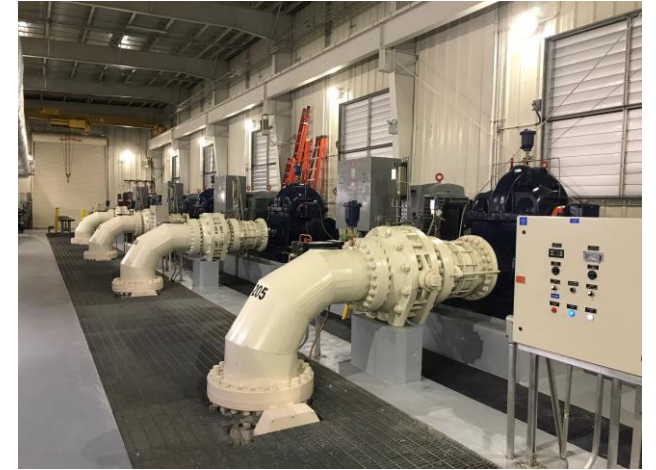
Woodsboro Pump Station
