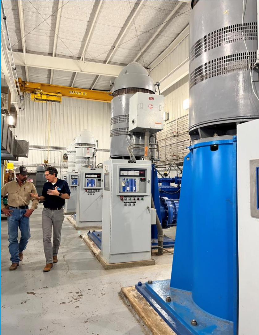
LNRA Intake Station
