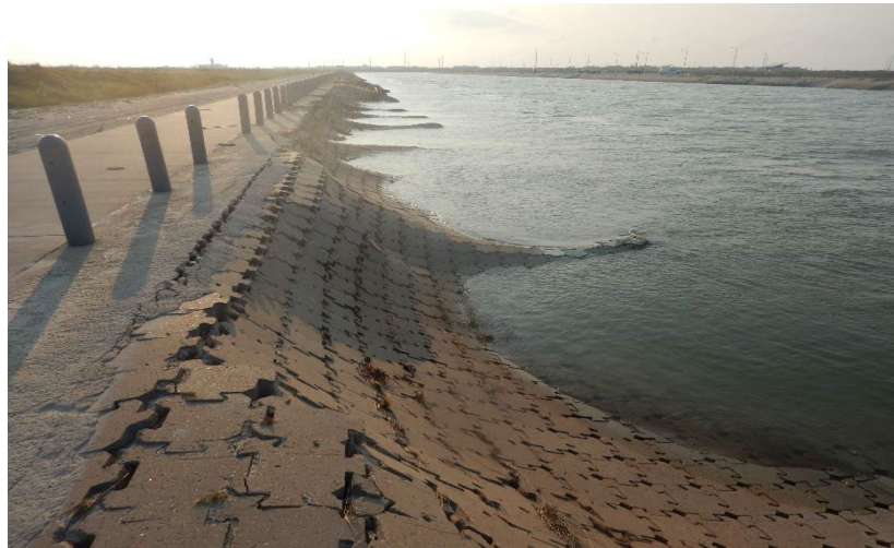
Figure 5 - Damages to ABM in Reach 3
