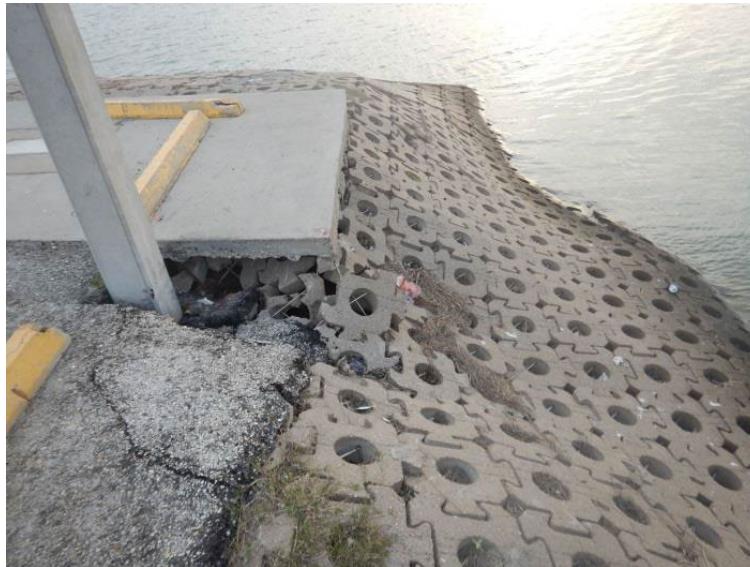
Figure 7 - Damages to ABM in Reach 4
