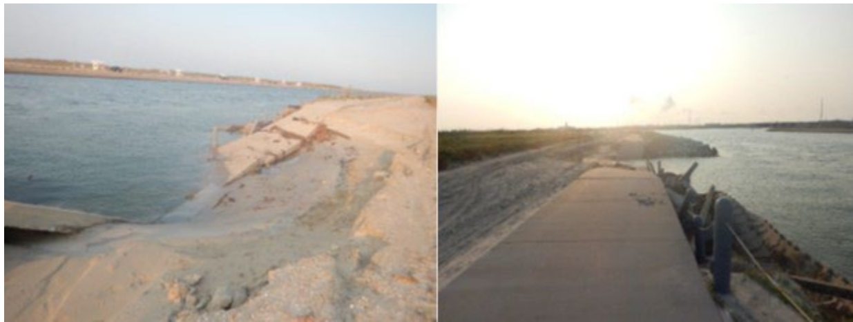
Figure 6 - Damages to Sidewalk in Reach 3
