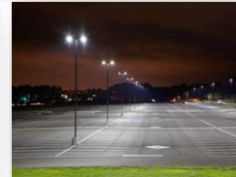
Example of Surface Lot Lighting
