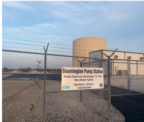
Bloomington Pump Station
