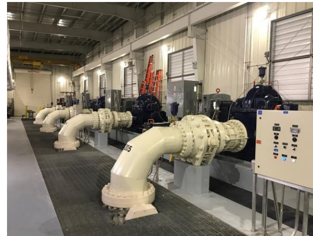
Woodsboro Pump Station
