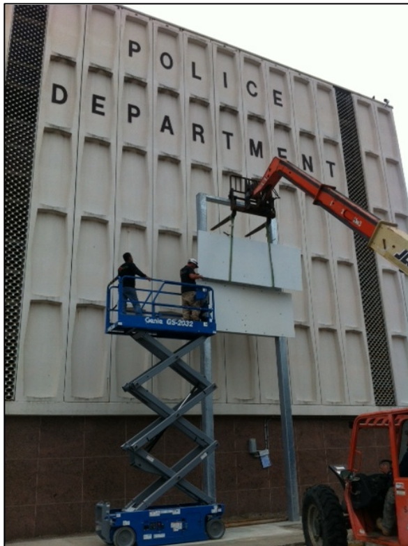
Installation of Free-Standing Wall for Jack Gron sculpture Police Department Building April 2013
