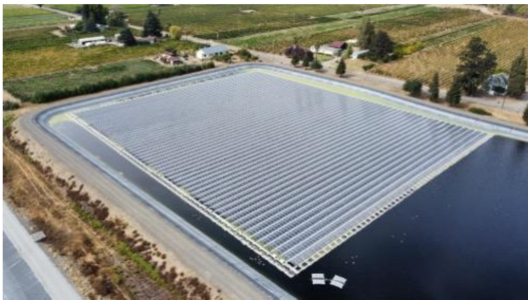
Largest FPV Project in the western hemisphere (when built, 2022)- 4.8 MW
